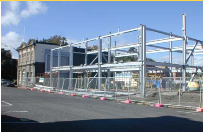
The new block steel frame goes up next to the older buildings.
